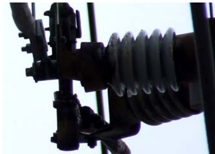
Failed switch with arc-damaged contacts
