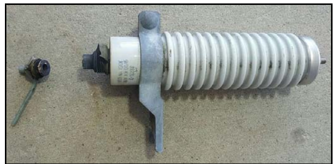
Fig. 9. Failed arrester associated with fault of Fig. 8
